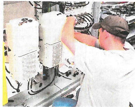
A Verizon technician completes the wiring of a small 5G cell. Verizon is rolling out the new technology in a number of U.S. cities, including Syracuse. Verizon Wireless
